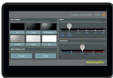
the touchpanel can provide integrated user control of lighting scenes, blinds, temperature and other services
